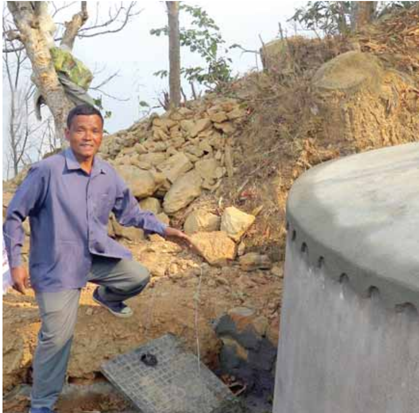
Mr. Prabhu Ram Pahari showing the reservoir tank and intake and outflow chamber.
