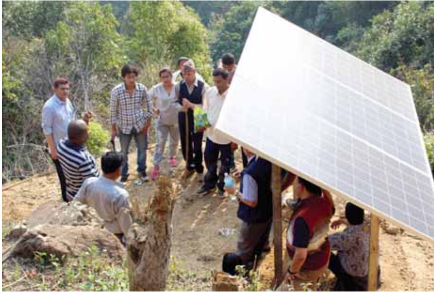
Saurya Bhanjyan Drinking Water Supply System (Hariharpur Gadhi, Sindhuli) uses solar powered pump to pump water from a low lying source to the main reservoir tank.
